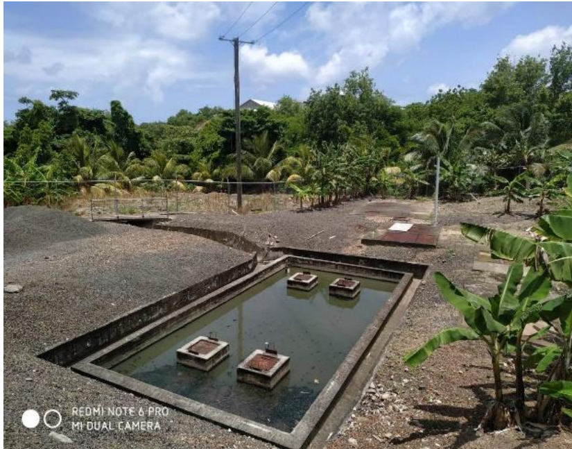
Existing Treatment Plant
