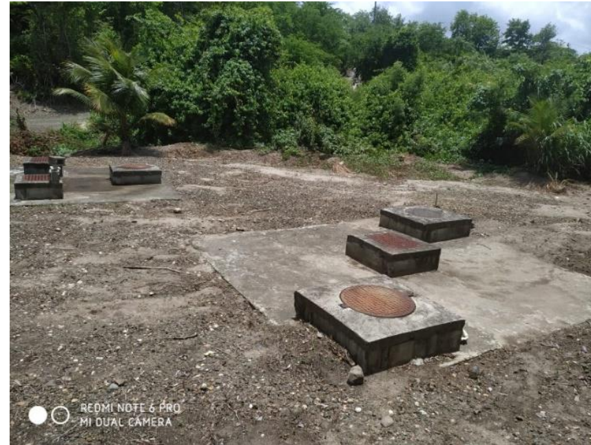
Black Bay - Series of 2 septic tanks
